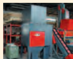
Dust collector for all materials
